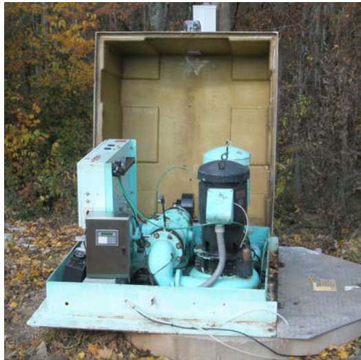
This is a picture of the AWS Dosing system installed inside the Sugar Tree #1 pumping station in Clarksville, TN.
